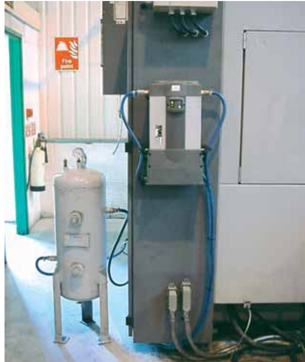
PNEUDRI MiDAS installed to supply control air for a CNC machining center
